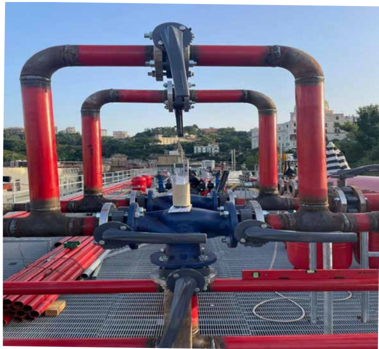
General view of the installation
